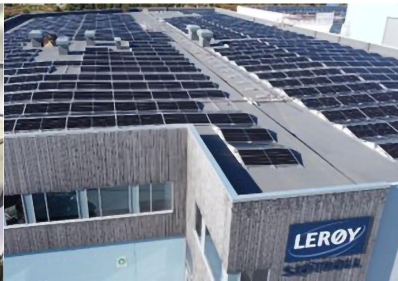
Solar panels at Kjærelva
