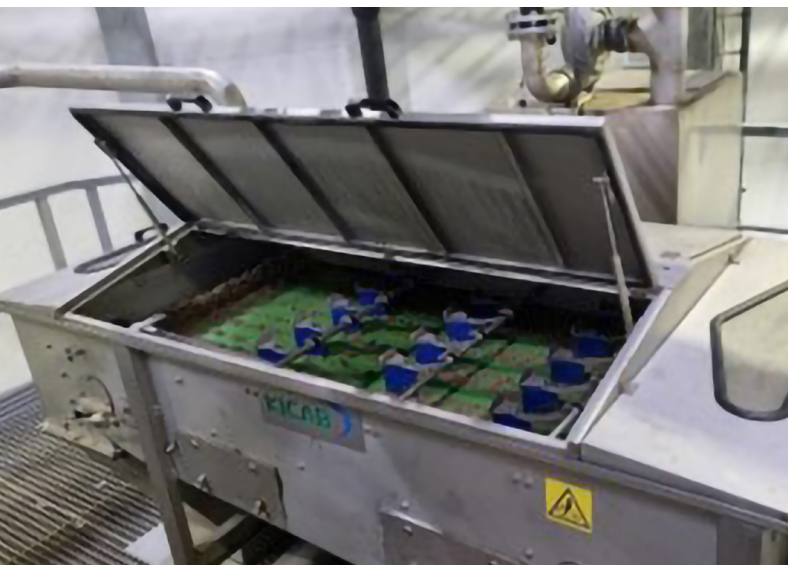
Sludge processing unit at Kjærelva
